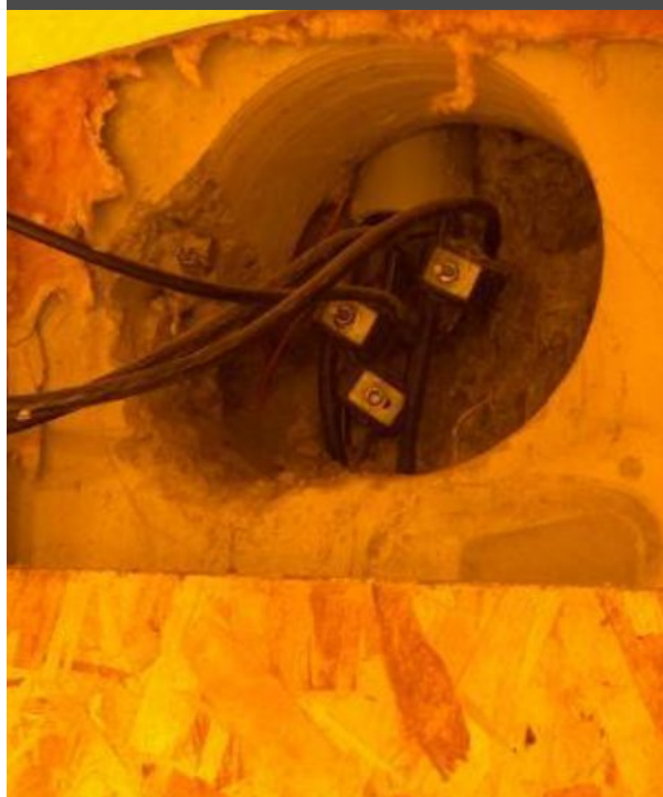
Figure 101. Illegally Diverted Electricity at an Indoor Marijuana Grow.
