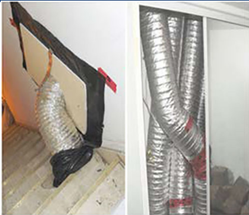
FIGURE 2. DO-IT-YOURSELF VENTILATION IN A COLORADO GROW HOUSE
